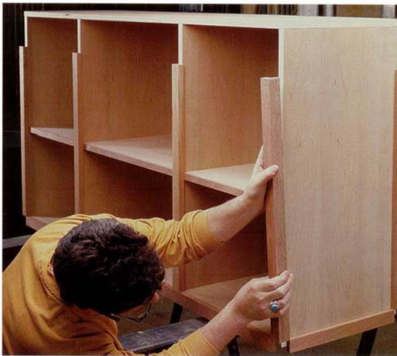
Photo A: Attach the corner piece of the face frame \frac{3}{4} in. shy of the bottom. This leaves a space for the corner block.
