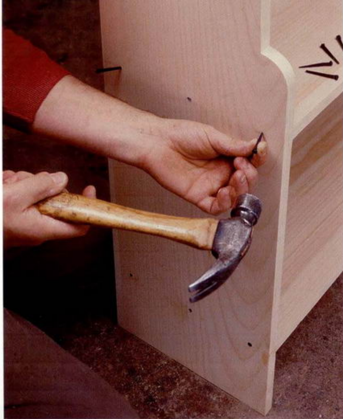
Photo C: Alternate the angle of the nails into the shelf ends to give the joint greater strength and to prevent them from pulling apart.
